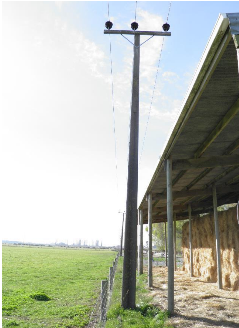
Shed close to lines – 11,000V
