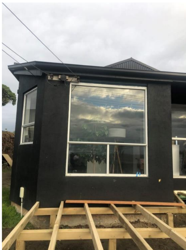
Deck built in close proximity to overhead service mains. From the finished deck the lines could likely be reached by those standing on it.
