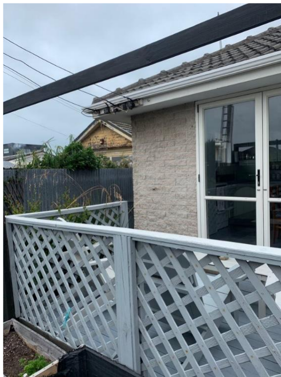
Fence, decking area and pergola located very close to the overhead service main.
