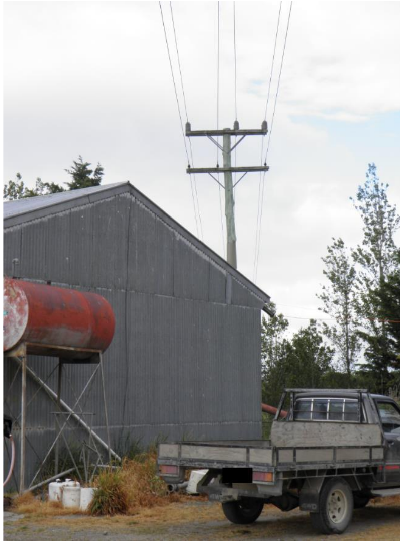
Shed under lines – underbuild– 11,000V
