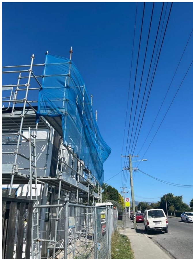
Scaffolding within the ECP:34 setback distances from low and high voltage lines (11kV)
