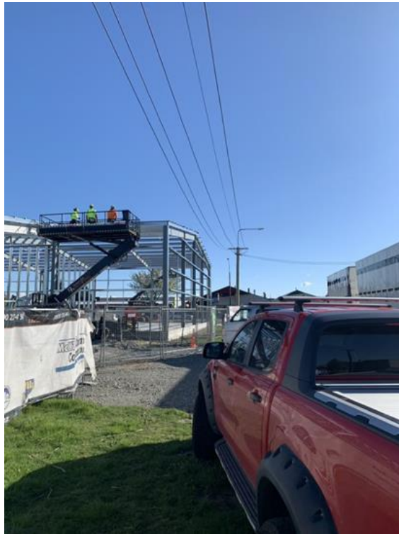
New development located in close proximity to the existing 400kV lines.
