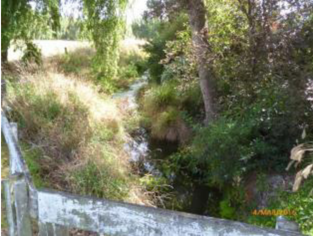
Woods Drain. Water levels are virtually flat along Woods Drain and Stackwoods Drain
