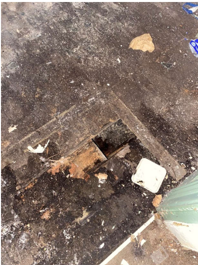
Fire damage to floor
