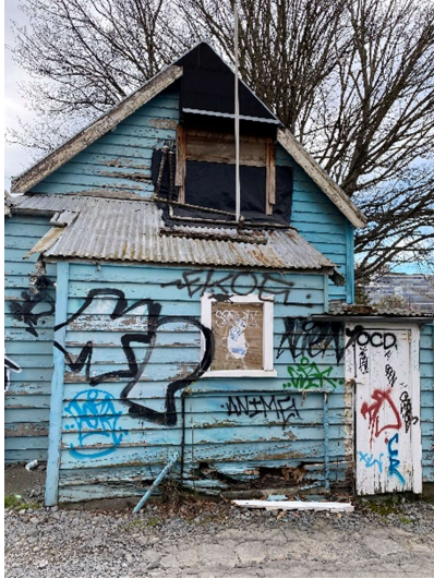
West Elevation (1 st gable end where chimney collapsed in earthquake)
