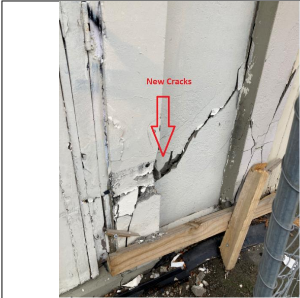
Photo 7 – View of new cracks at East wall
