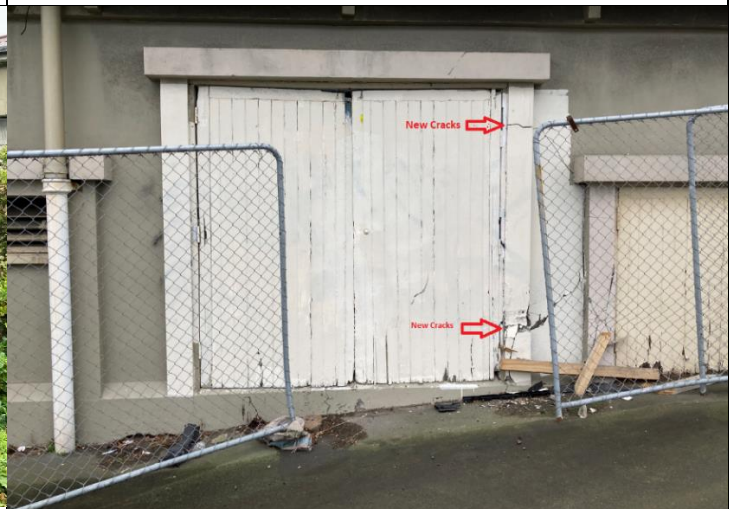
Photo 6 – View from East wall with new cracks.
