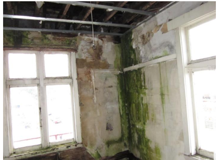
Damaged ceilings, walls/ mould /moisture and weather penetration damage
