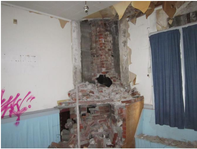
Broken & damaged fireplace
