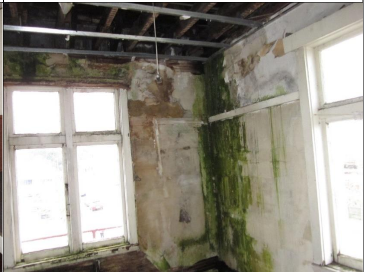
Photo 12 – View form interior – Visible water damaged on the roof and wall
