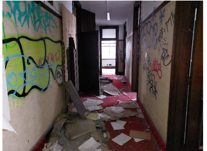
Photo 20: Evidence of condition – Second Floor Hallway
