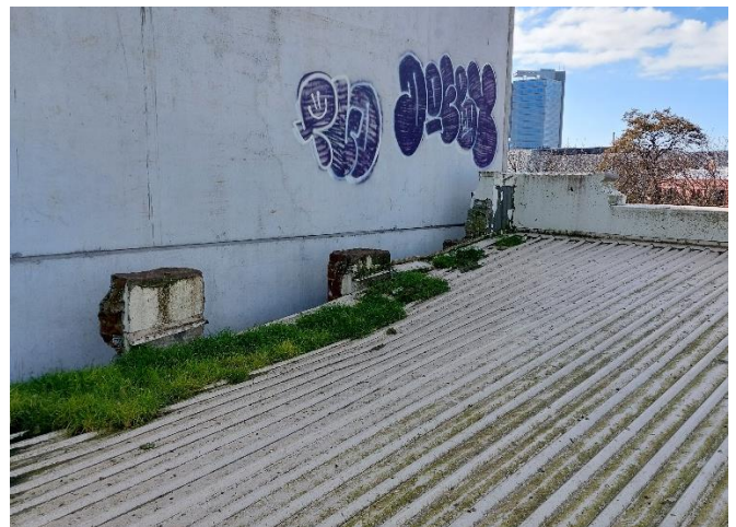
Photo 30: Evidence of condition - Roof to northern section of building
