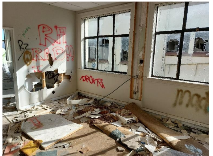
Photo 22: Evidence of condition –Room 30
