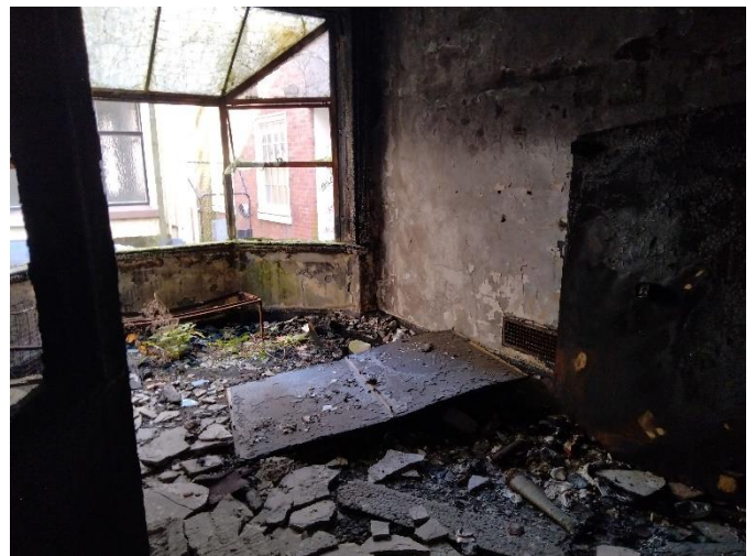
Photo 12: Evidence of condition – Fire damaged parts of Room 1
