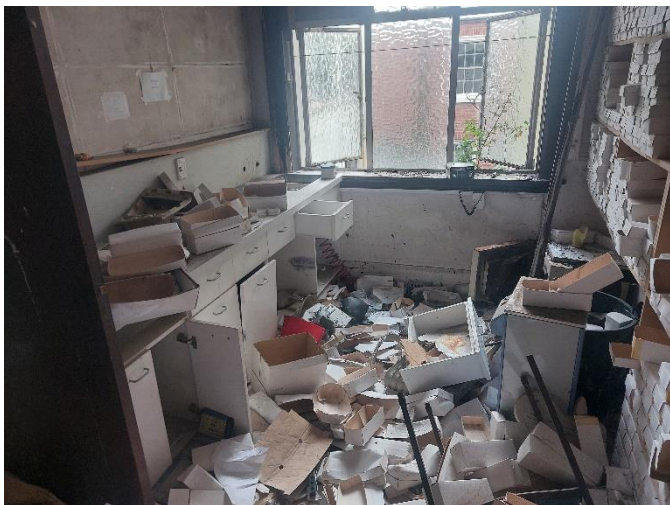
Photo 17: Evidence of condition – Room 20
