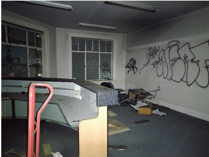
Photo 7: Evidence of condition – Room 5
