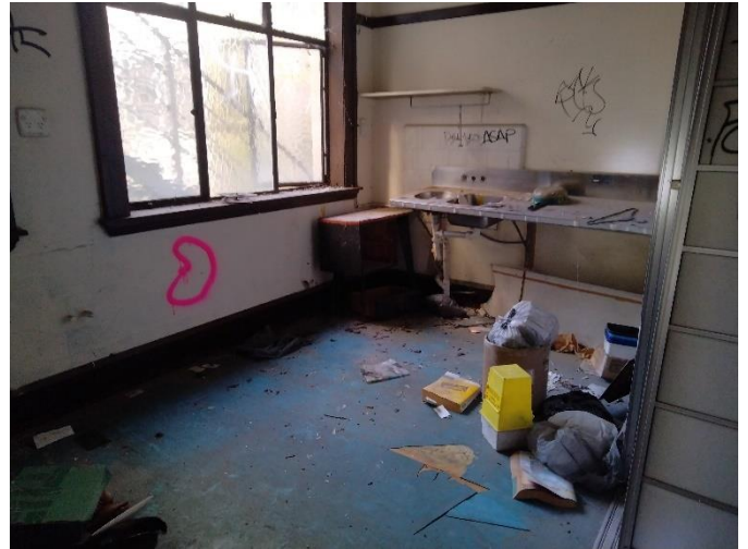
Photo 8: Evidence of condition – Room 9
