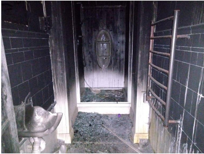
Photo 13: Evidence of condition – Fire damaged parts of Room 1
