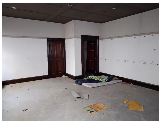
Photo 6: Evidence of condition – Room 8
