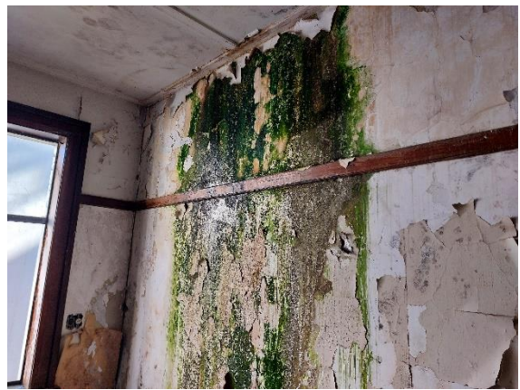
Photo 17: Water damaged area (L2 Room 9)
