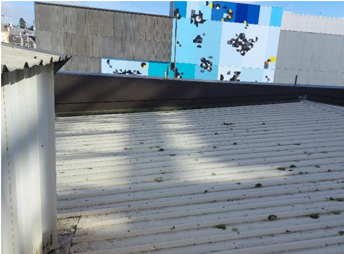
Photo 27: Evidence of condition - Roof to northern section of building
