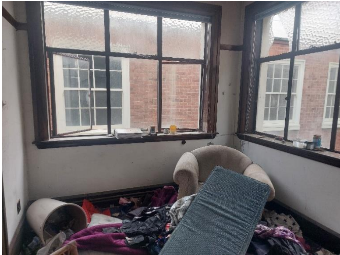
Photo 19: Evidence of condition – Room 19
