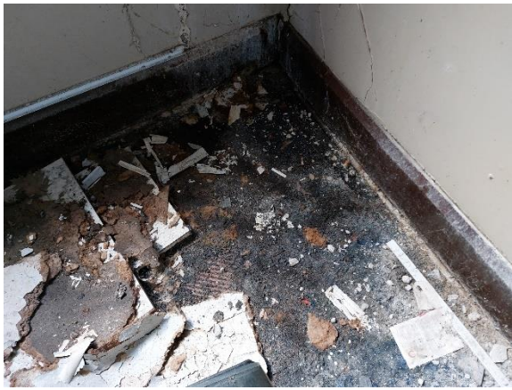
Photo 13: Water damaged area (GF Room 8)
