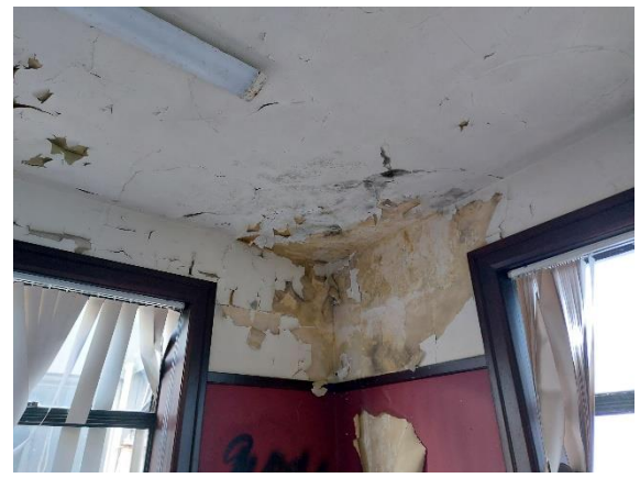
Photo 16: Water damaged area (L1 Room 11)
