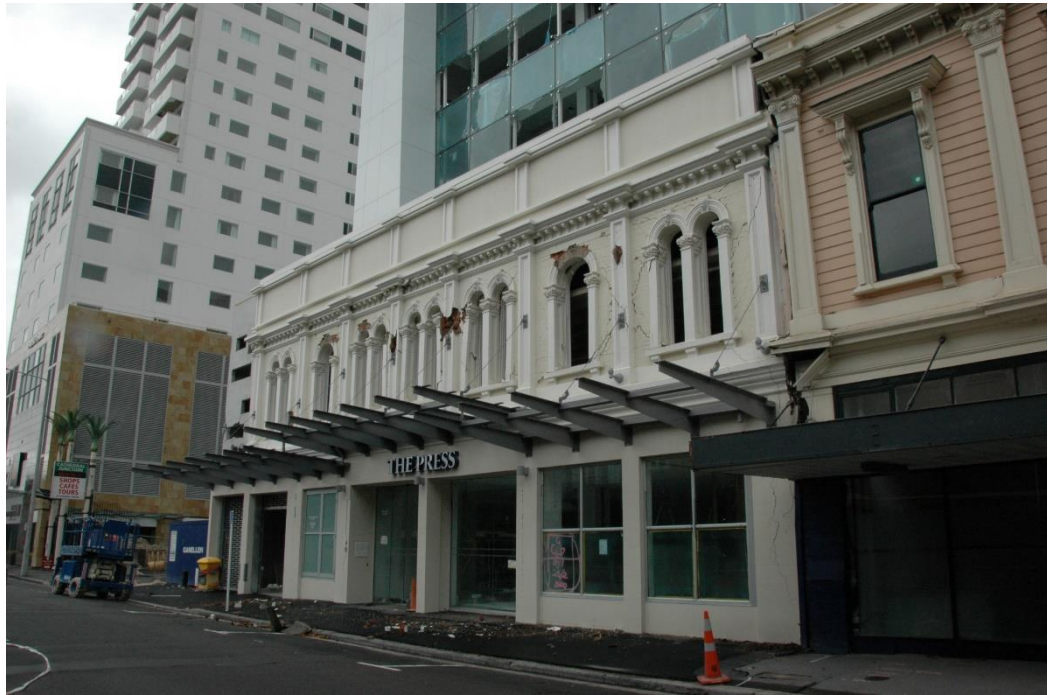
Photograph 2: 158 Gloucester Street, Christchurch – post February earthquake
