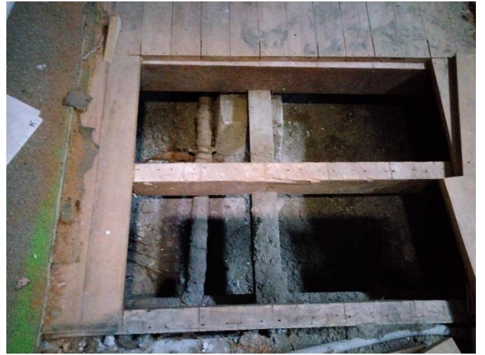
Photo 14: Limited access to Subfloor in Room 2
