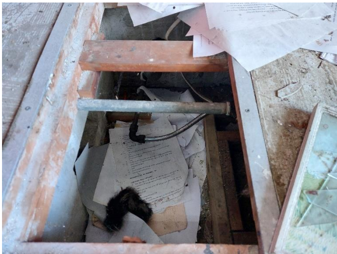
Photo 21: Evidence of condition – Floor space in Room 29
