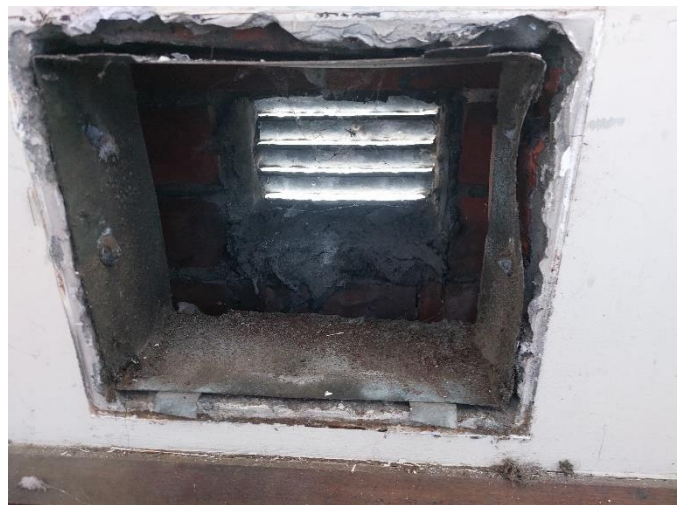
Photo 24: Evidence of condition – Vent to wall
