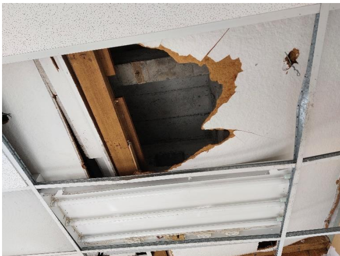
Photo 23: Evidence of condition – Room 30 ceilings
