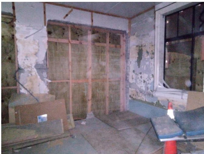
Photo 11: Evidence of condition – Room 3
