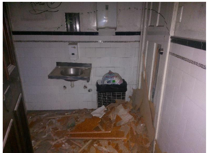
Photo 18: Evidence of condition – First Floor Ladies W/C
