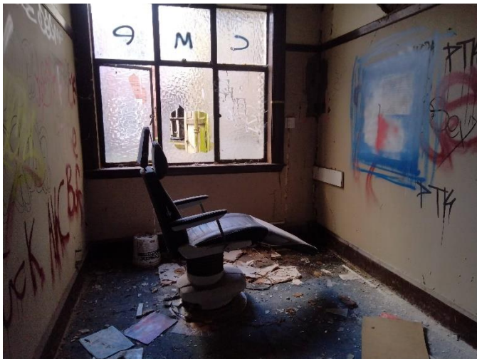
Photo 9: Evidence of condition – Room 9
