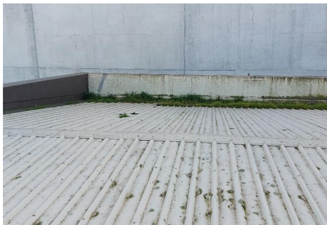
Photo 31: Evidence of condition – Roof to northern section of building
