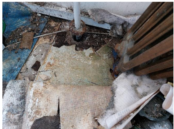
Photo 18: Water damaged area (L2 Room 29)
