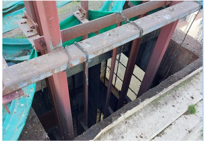
Photo 28: Evidence of condition - Top of lift shaft
