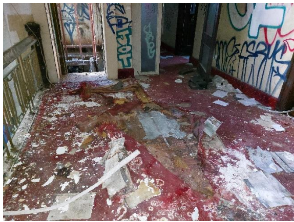
Photo 15: Evidence of condition (L1 Landing)
