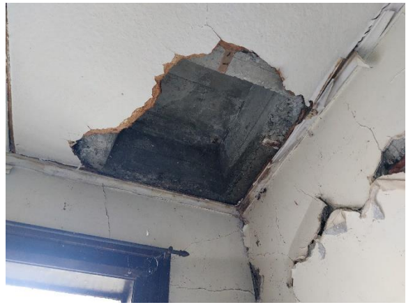
Photo 14: Example of structural damage
