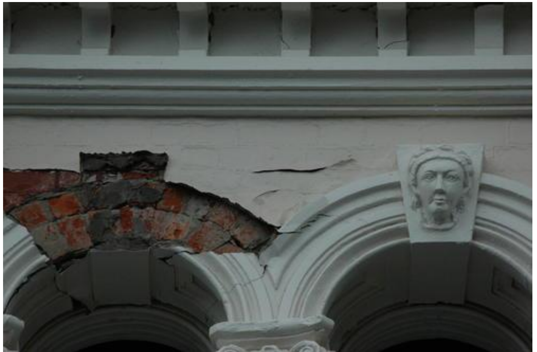
Photograph 3: 158 Gloucester Street, Christchurch – post February earthquake
