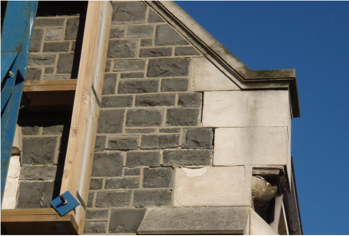
Photo 4 – Loose masonry and cracking on east gable wall, but random repair is required throughout the church walls and chancel arch
