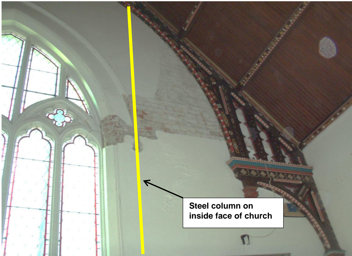
Photo 2b – Interior view of west gable showing render damage (masonry cracking exists but is not visible on this photo)
