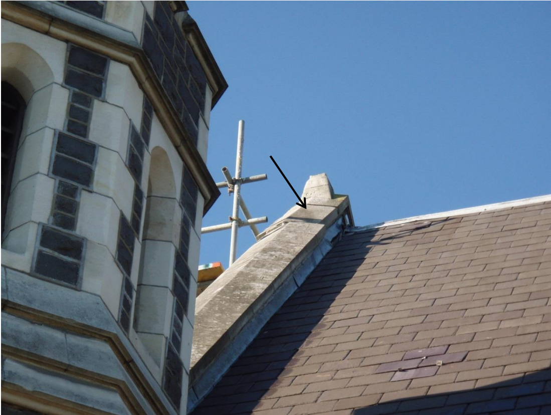
Photo 5 – Dislodged capping stones over chancel arch
