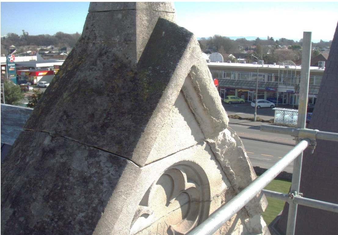
Photo 5a – Capping stone damage over chance arch
