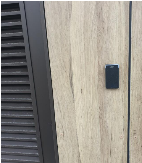
Cycle parking room 2: Access likewise via RFID reader.
