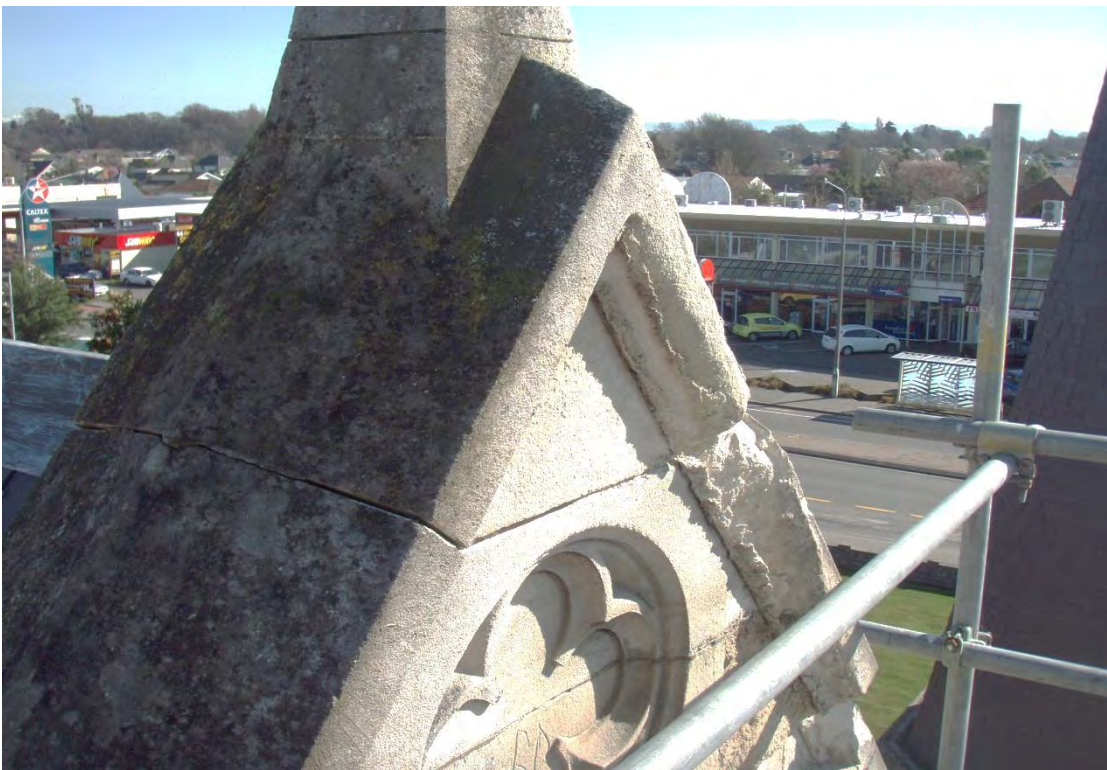
Photo 5a – Capping stone damage over chance arch
