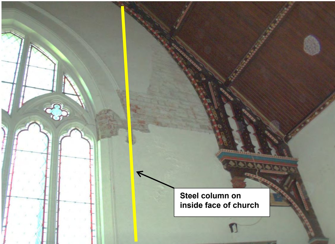
Photo 2b – Interior view of west gable showing render damage (masonry cracking exists but is not visible on this photo)
