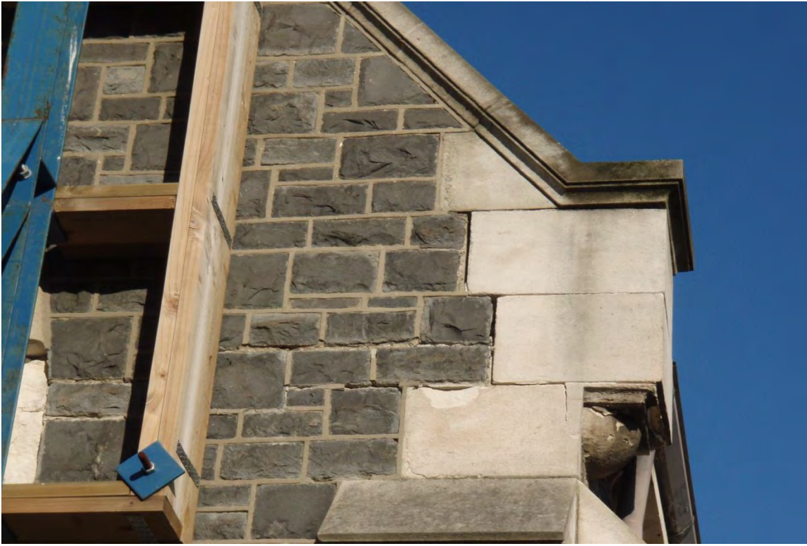
Photo 4 – Loose masonry and cracking on east gable wall, but random repair is required throughout the church walls and chancel arch
