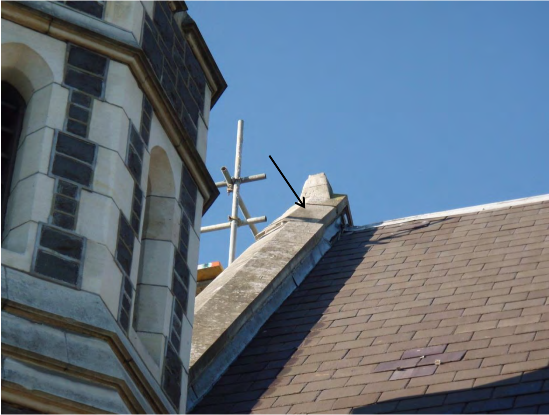
Photo 5 – Dislodged capping stones over chancel arch
