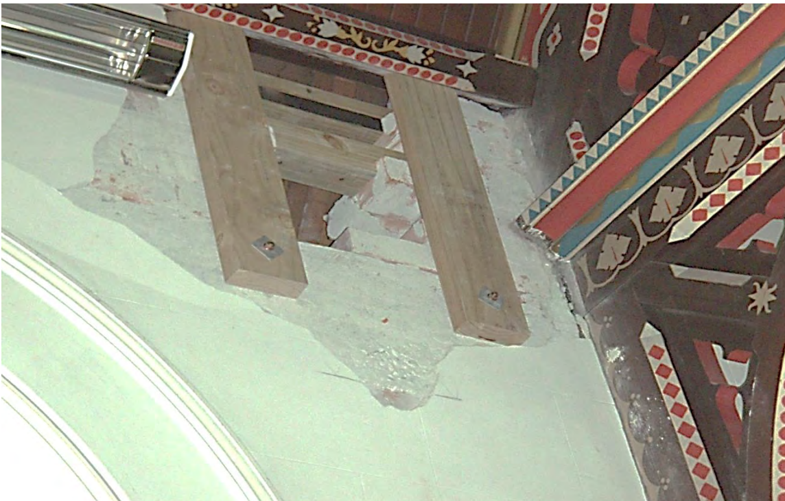
Photo 3a – brick work along top of side walls (opened for investigation purposes)
