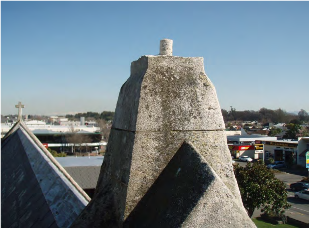
Photo 5b – view at roof level looking from chance arch (cross support will need stitching)
