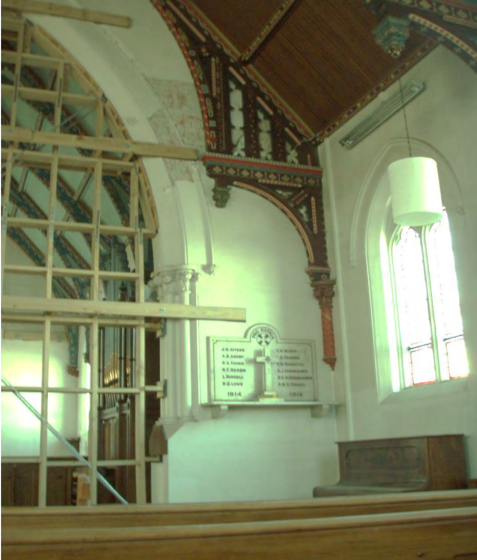
Photo 1a – Chancel arch, render damage and cracking at nave wall eave level
