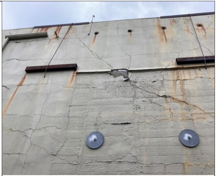
Photo 8 – View of concrete spalling at West wall (in close proximity to the neighbor driveway)
