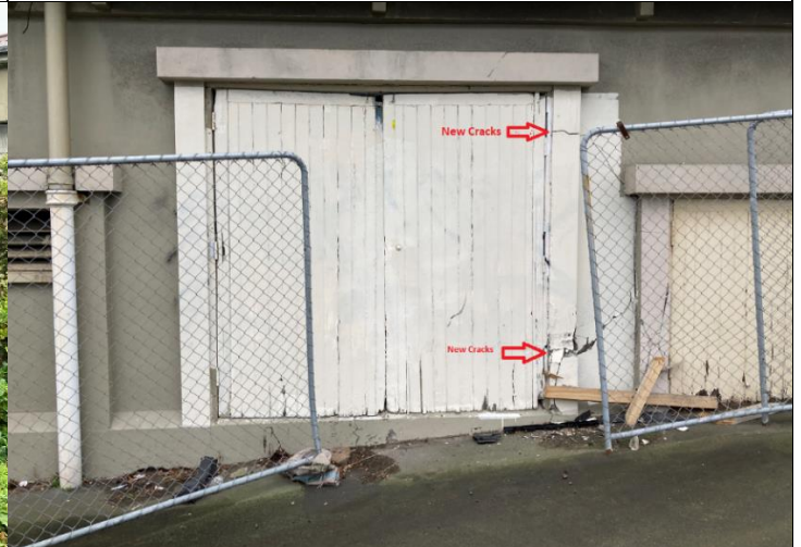
Photo 6 – View from East wall with new cracks.
