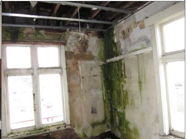
Photo 12 – View from interior – Visible water damaged on the roof and wall
