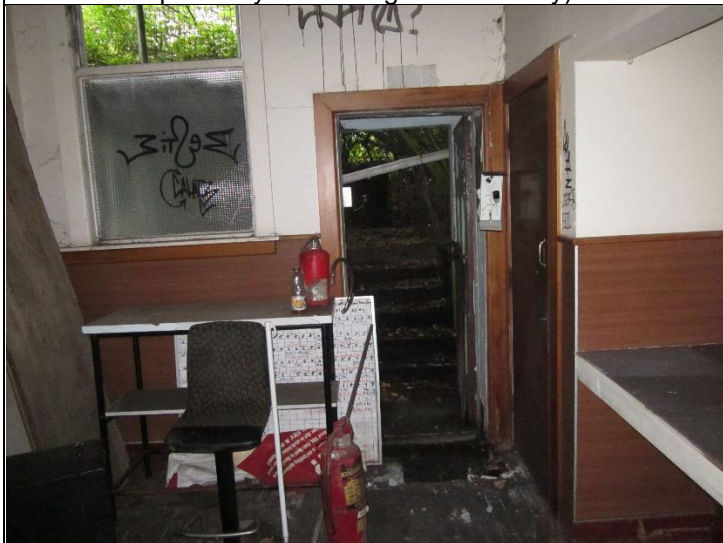
Photo 11 – View from interior. Another access to rear part of the building. It would appear the building had been assessed by others.
