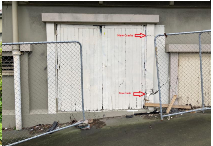
Photo 6 – View from East wall with new cracks.
