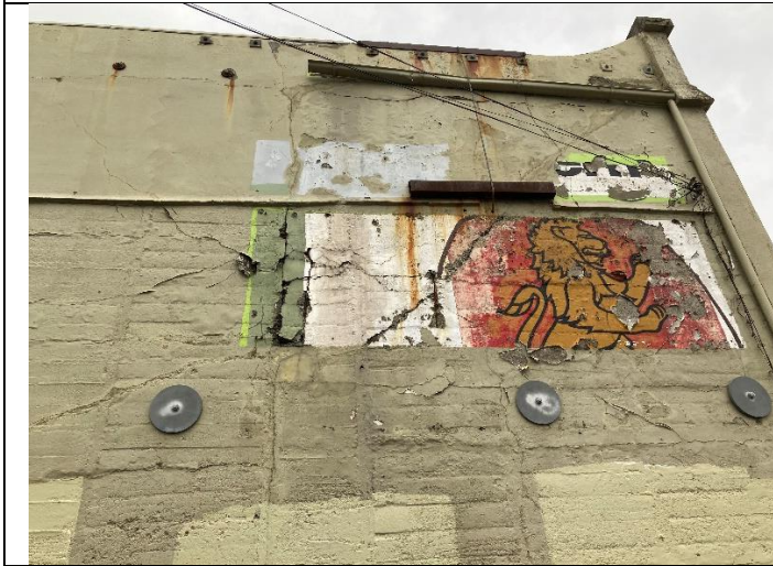
Photo 9 – View of concrete spalling at West wall (in close proximity to the neighbor driveway)
