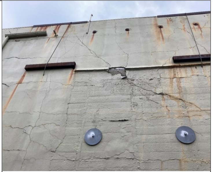
Photo 8 – View of concrete spalling at West wall (in close proximity to the neighbor driveway)
