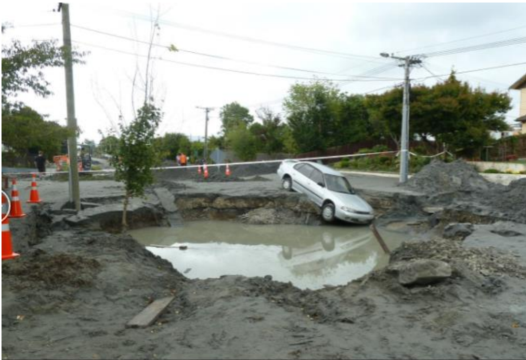
Road damage caused by broken pipe
