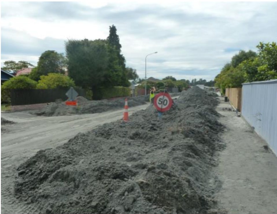
Liquefaction ejecta piles along street
