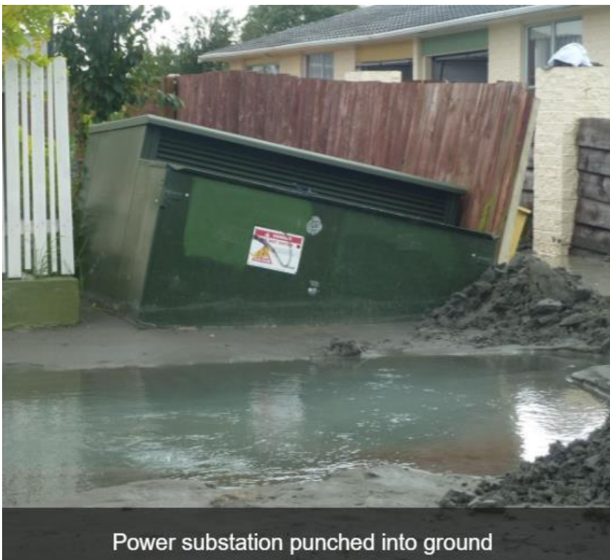
Lateral spreading damage to power lines
